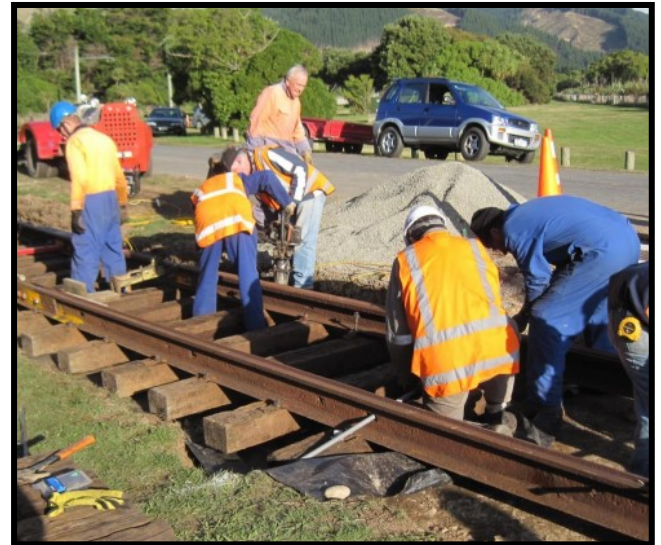
A team of Tramway Museum volunteers on 10th June, preparing tram tracks for a new road crossing in Queen Elizabeth Park
